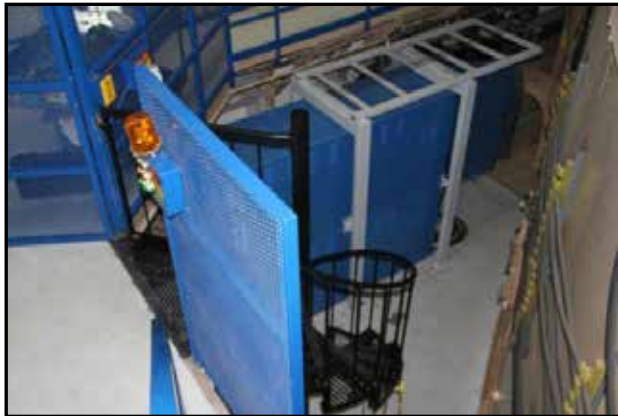
Capacitor bank system on Z 900 kJ, 8 mF, 15 kV (Feb. 2013)
